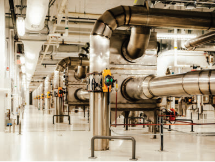
A HEPA system filters all exhausted air from the Level 3 facility before it's released.
